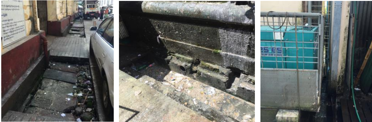
Figure 22 - Open drains in 39th street pose a health & safety risk, while generators block pedestrian access
