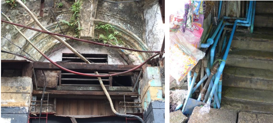
Figure 24 - Haphazard installation of water and electricity supply pipes
