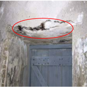
Cracks in walls of upper terraces
